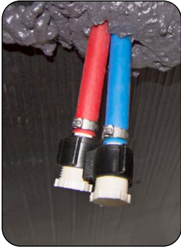
Low-Point Drain Valves located under the RV
