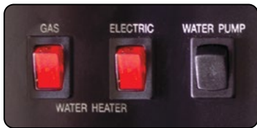
Water Pump & Water Heater On/Off Switches
