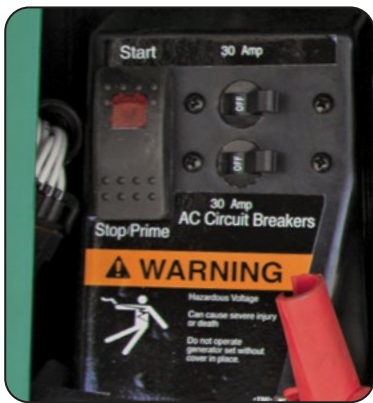
Generator main power & circuit breaker switches.
