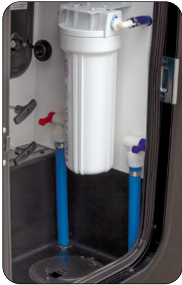
Low-Point Drains and Water Filter (if equipped) are located with the Universal Docking Station
