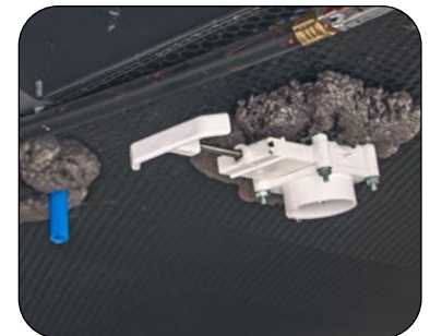
The Fresh Water Holding Tank Gate Valve is located under the RV
