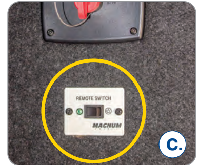
Inverter Remote Switch
