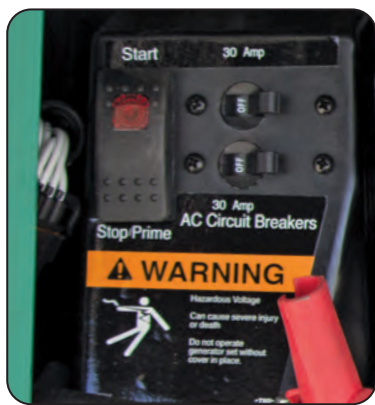
Generator main power & circuit breaker switches.
