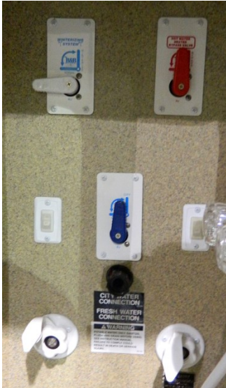
Typical valve positions for sanitization (connect hose to white city water fill inlet, located to the left of the white sewer tank flusher water inlet).
