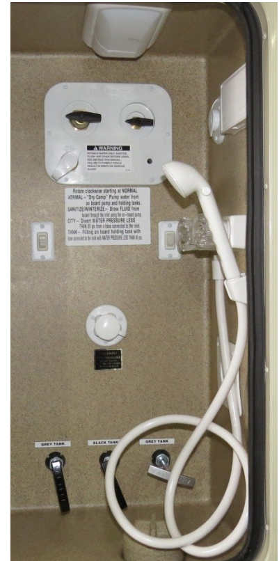
Photo above shows a typical utility center with the “Anderson Kantleak” installed.
