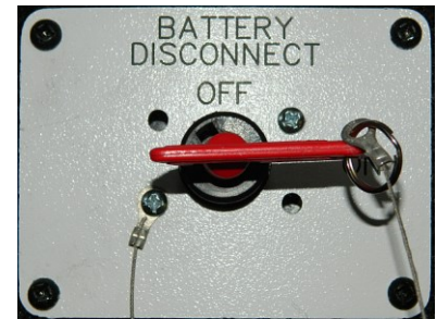
Typical battery disconnect switch
