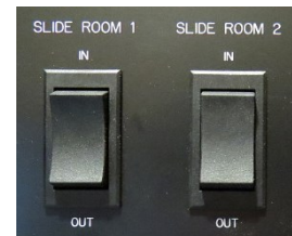
Typical slide room switches, located in the Command Center
