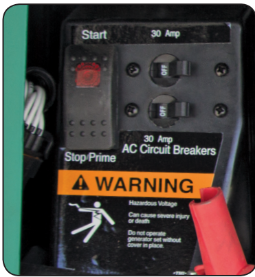
Generator main power & circuit breaker switches.
