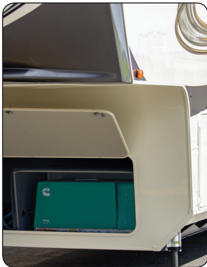
Generator (if so equipped) is located in the front compartment of your RV.
