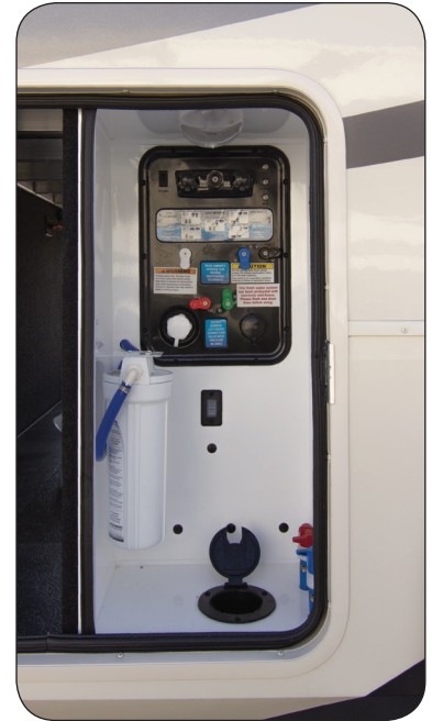
The Nautilus P1 System Is Located in the Exterior Docking Station
