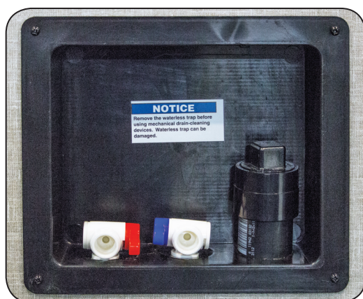
Hot & Cold Water Washer Hookups are typically located in the kitchen.
