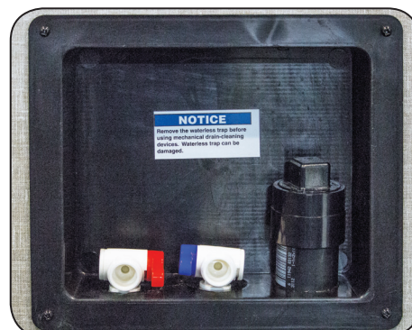
Hot & Cold Water Washer Hookups are typically located in the front bedroom or in the rear garage area.
