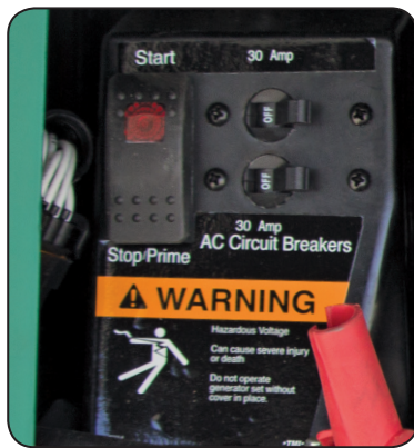
Generator main power & circuit breaker switches.
