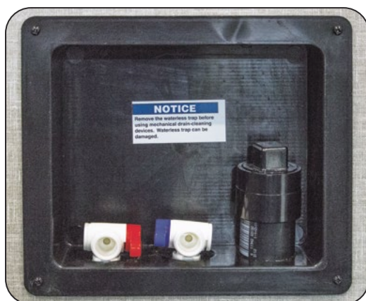
Hot & Cold Water Washer Hookups
