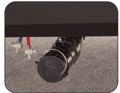
Sewer Outlet Connection Is Located Under the RV on the Off-Door Side
