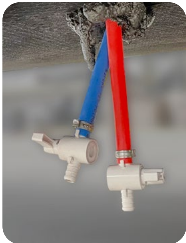
Low-Point Drains located under the RV
