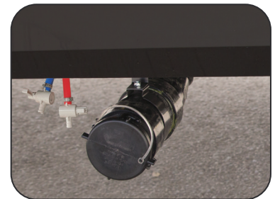
Sewer Outlet Connection Is Located Under the RV on the Off-Door Side
