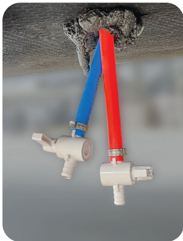
Low-Point Drains located under the RV
