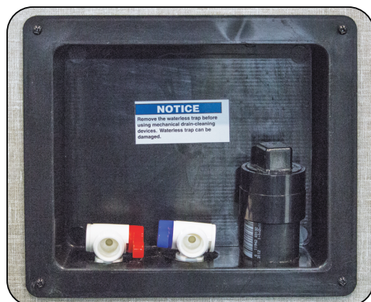
Hot & Cold Water Washer Hookups
