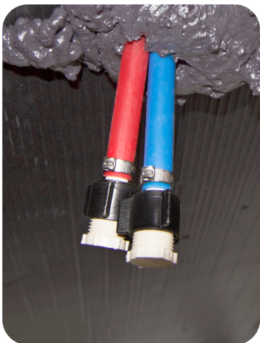
Low-Point Drains located under the RV
