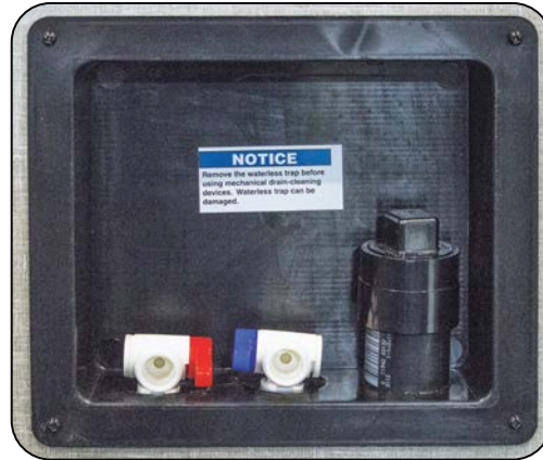
Hot & Cold Water Washer Hookups
