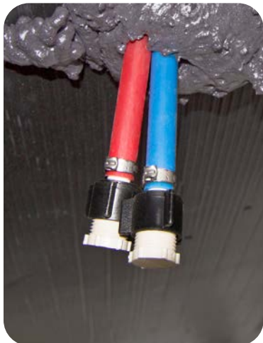
Low-Point Drains located under the RV
