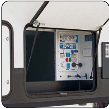
The Nautilus P1 Water Control System Is Located On The Forward Off-Door Side.
