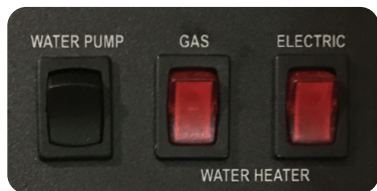
Water Pump & Water Heater On/Off Switches
