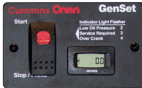
Generator Remote switch is found on the Command Center
