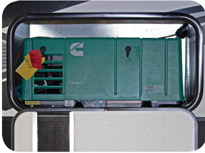
Generator (If So Equipped) Is Located in the Forward Off-Door Side Compartment of Your RV.
