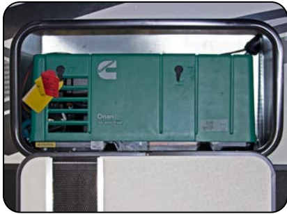
Generator (If So Equipped) Is Located in the Forward, Off-Door Side Compartment of the RV.
