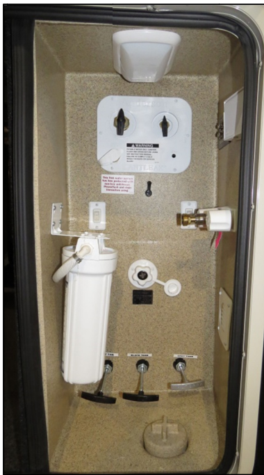
Close-up of a typical utility center.
