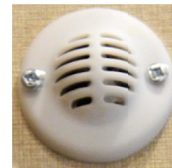
Typical temperature sensor (wall-mounted).
