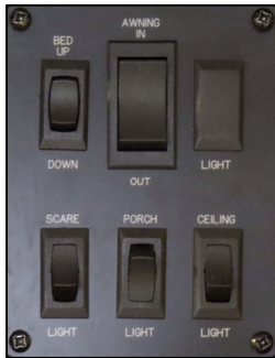
Typical Mini-Command Center, located in the garage area.
