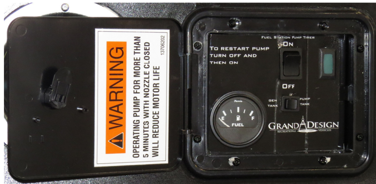
Typical fuel dispensing system emergency shut off switch hatch
