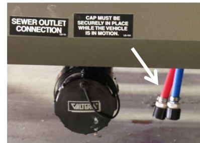
The white arrow indicates the blue and red colored low point drain lines.
